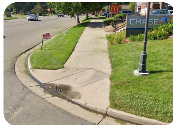
Non-compliant curb ramp at King Soopers driveway
